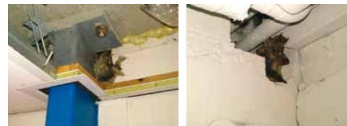
Contaminated insulation material found inside hidden structural elements.
